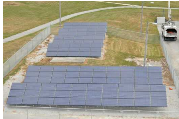
BMU Solar Lease: ~ 60 kW
